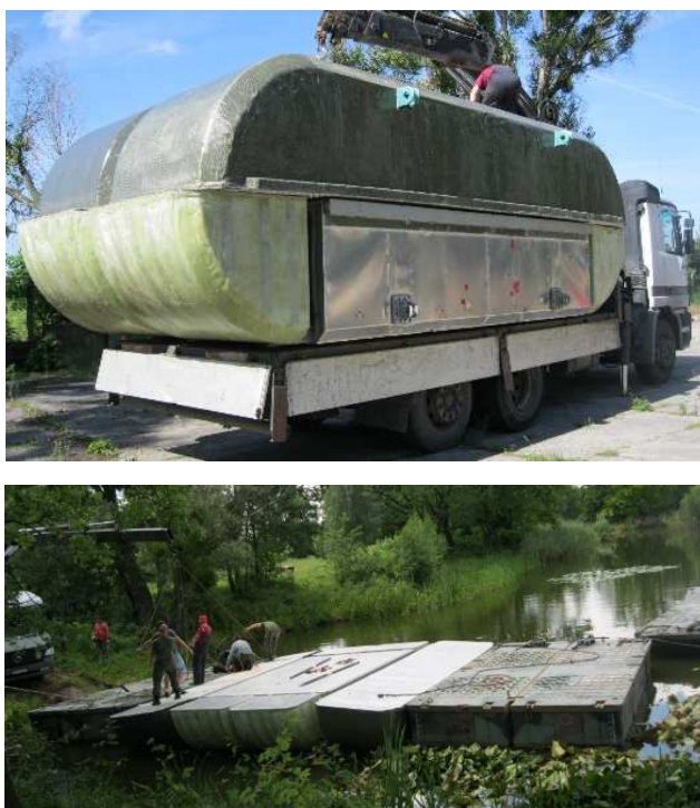
Fig. 6. Segment transport and construction of the crossing in combination with PP-64 segments
