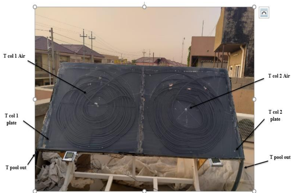
Fig. 6. Solar collector and thermocouple sensor location.
