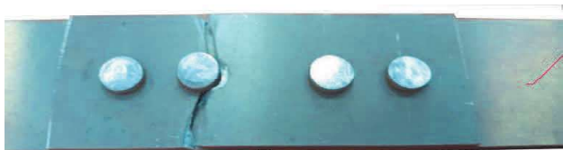
Fig. 11. Fatigue crack of flat cover plate
