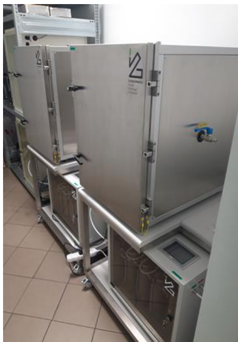
Fig. 11. View of implemented VOC emission test chambers
