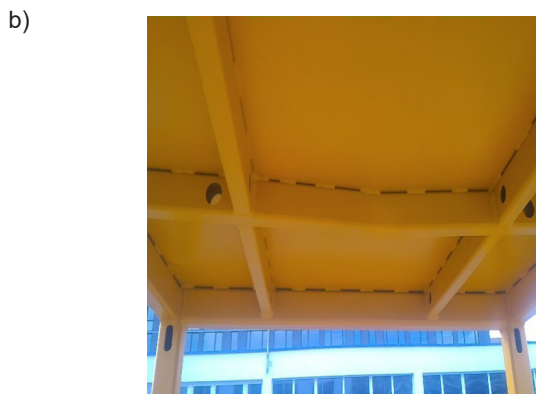
Fig. 15. FOPS structure under test procedure (a) and roof deformation after impact load (b)
